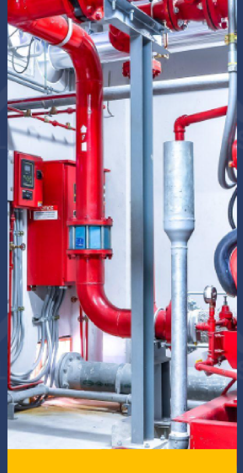
FIRE FIGHTING SYSTEM
